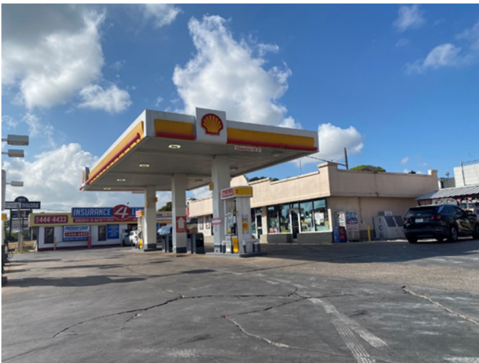
Photo 3: Map ID 476, a High Risk site. Photograph was taken from the corner of E. Riverside Drive, facing east.
