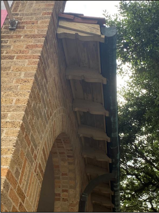
Detail view of the carved rafter ends and copper gutters on the 1926 section of the building.
