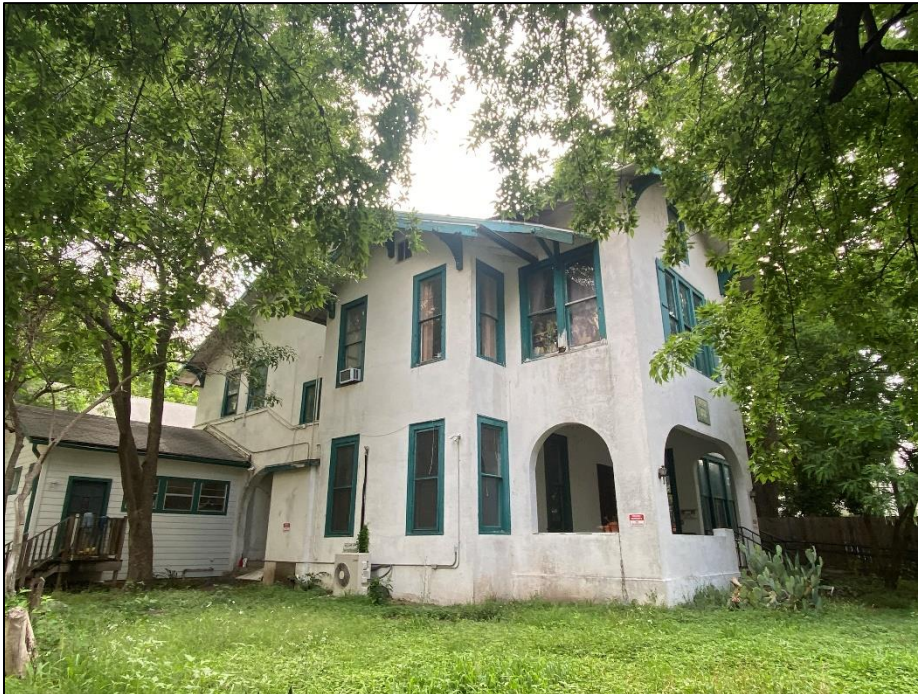
Oblique view of the façade and the west elevation of Resource S159, looking northeast.
