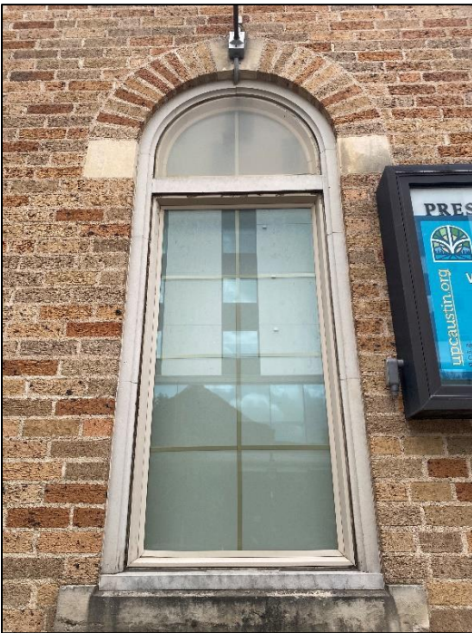
Detail of a replacement window on the west elevation of the 1926 building.
