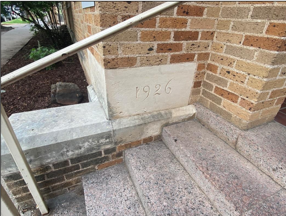
Detail of the stairs and cornerstone to the 1926 section of the building, looking north.
