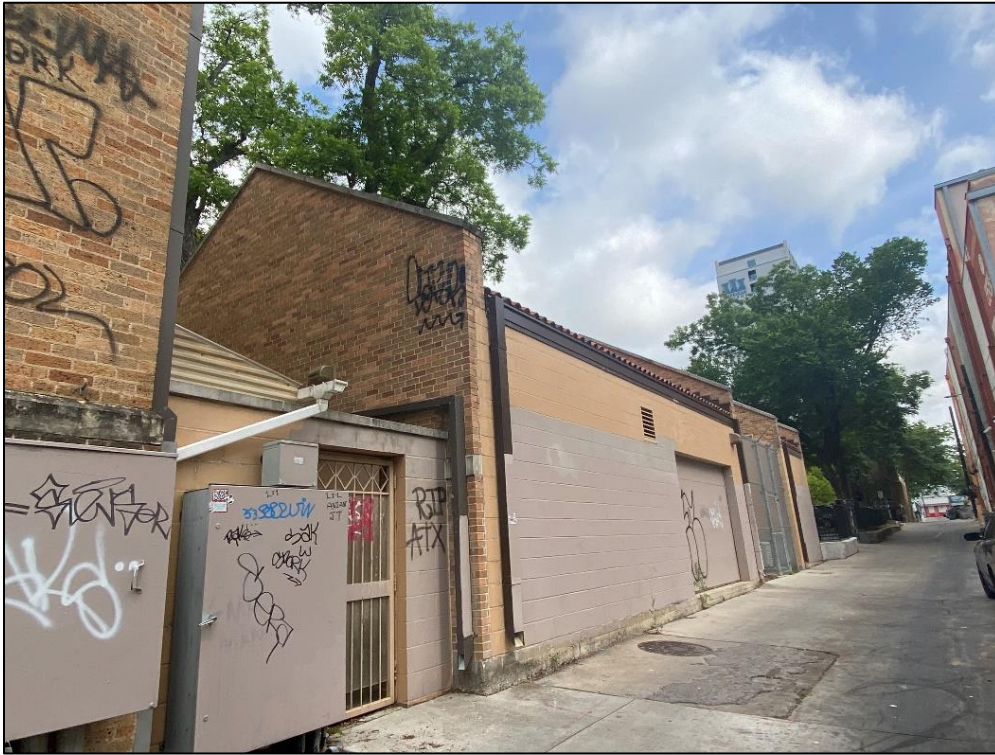
View of the east (rear) elevation of Resource S162, looking northwest (IMG_1523).
