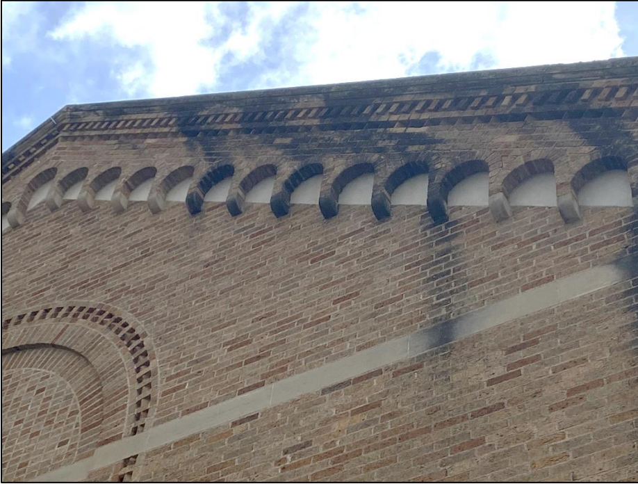
Detail of the brickwork along the cornice of the west elevation of the 1926 section of the building.
