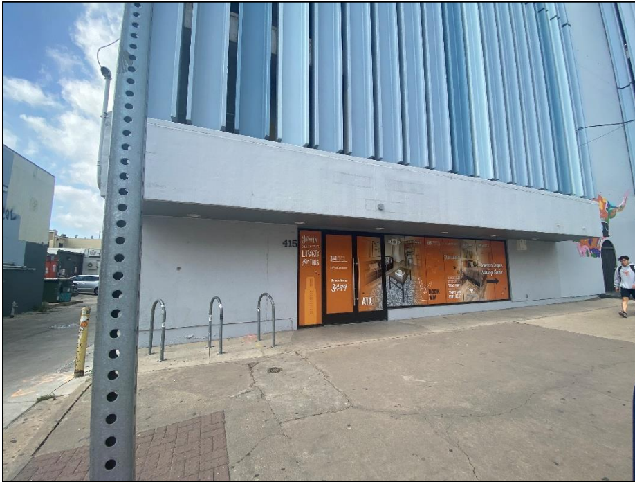
View of the lower level of the north elevation, looking south (IMG_1553).
