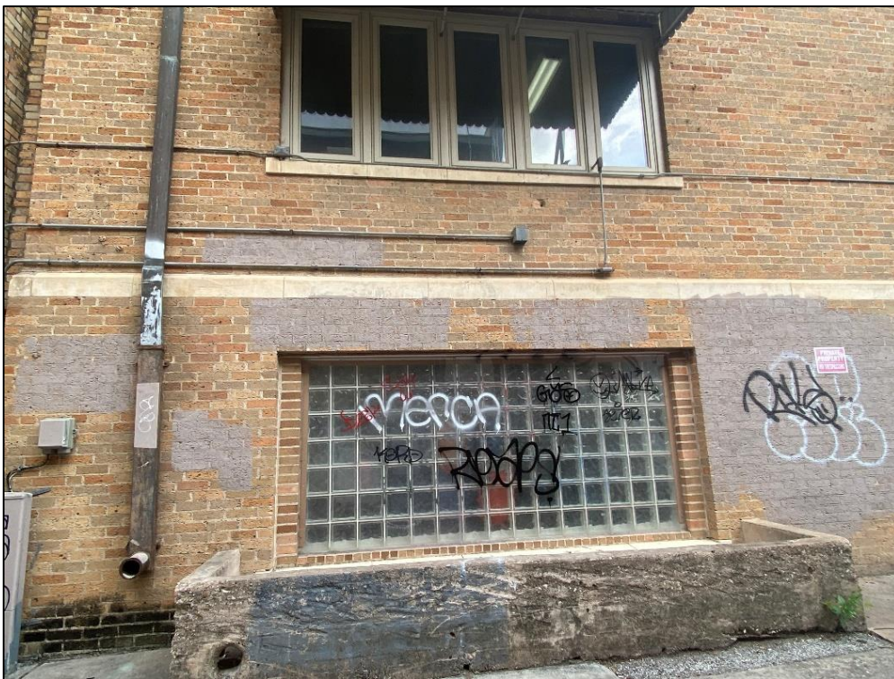
Detail view of a basement window on the east elevation of the 1926 building of Resource S162, looking west.
