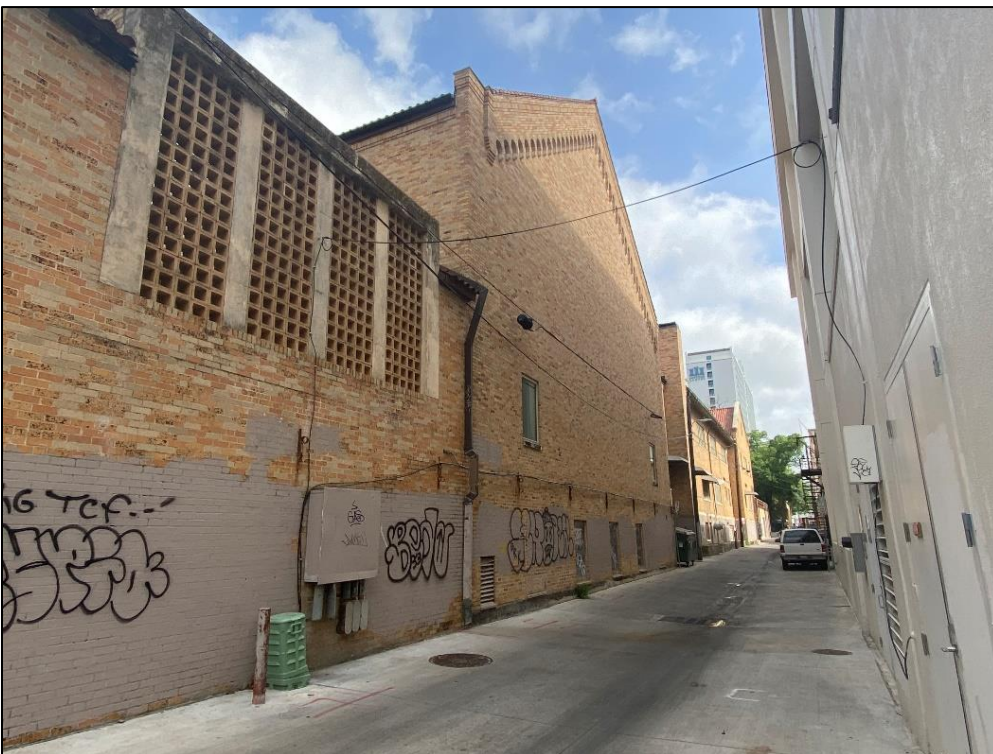
View of the east elevation of the 1926 and 1953 sections of Resource S162, looking north.
