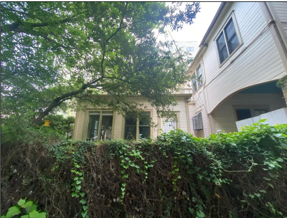
View of the south elevation of the rear (west) addition and the rear (west) elevations of the main block and the southern addition, Resource S148, looking north.
