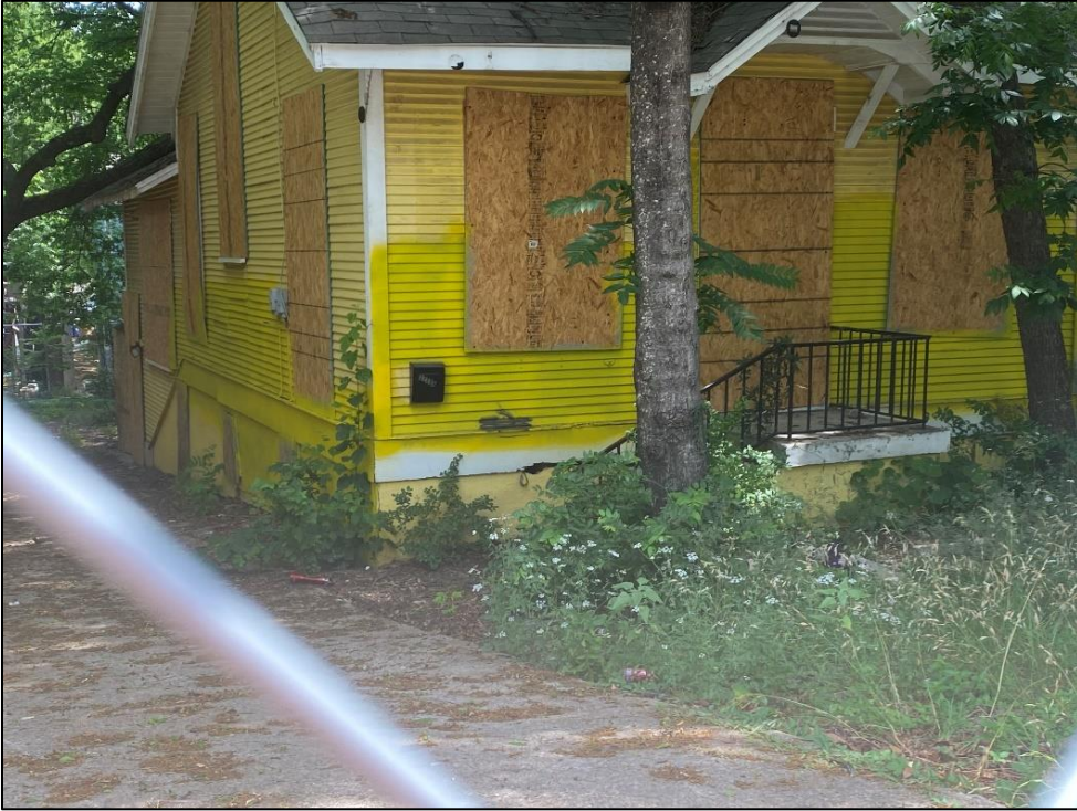
Oblique view of the north elevation and façade of Resource S137b, looking southeast.
