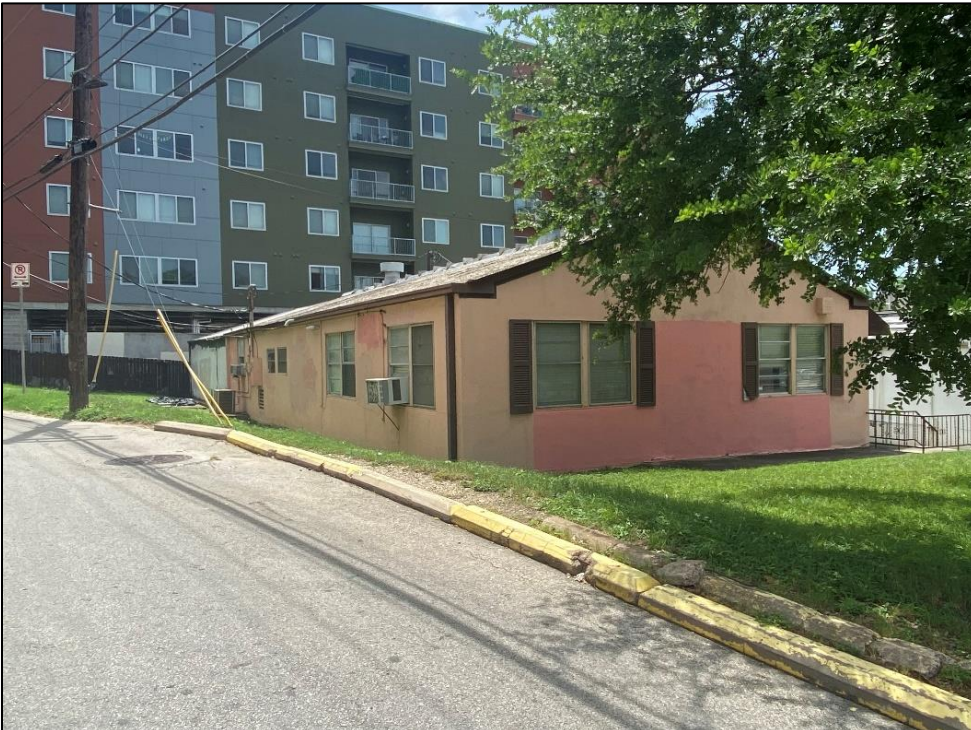
Oblique view of the rear (southeast) and northeast elevations of Resource S127b, looking southwest.
