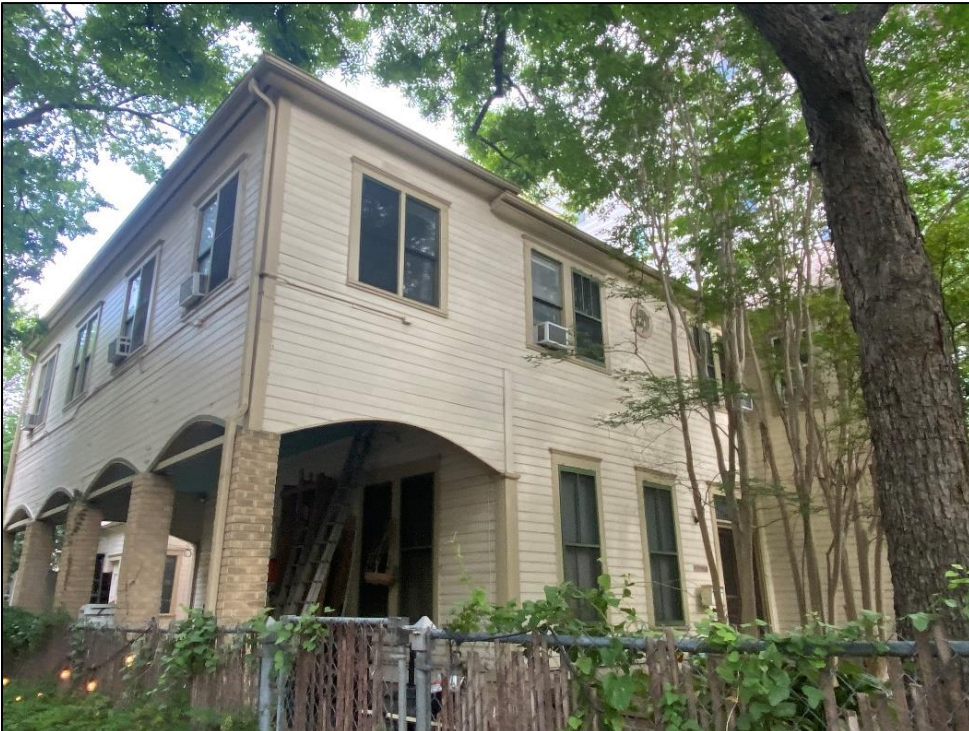
Oblique view of the south elevation and façade of Resource S148, looking northwest.
